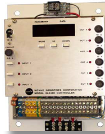
The sophisticated Novax Fire Hall Controller Unit is the heart of the system.
